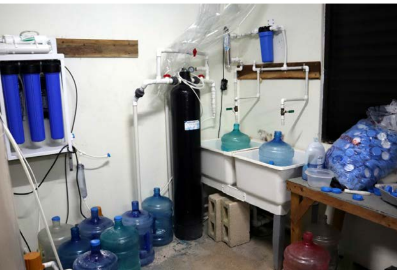
An interior view of the plant
